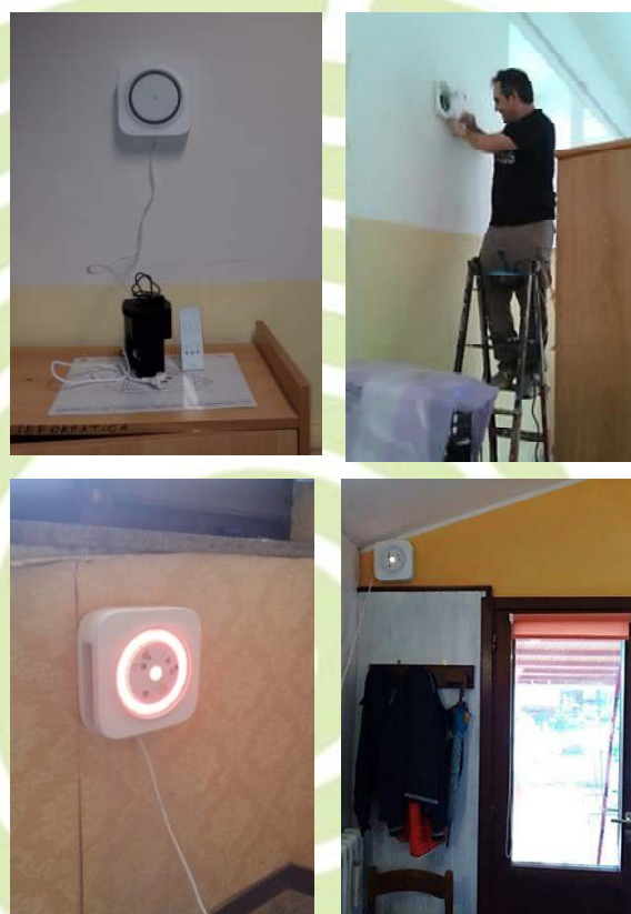
Figure 1. Photographs showing some installations of the fan and radon sensor.
